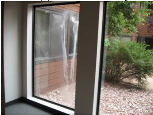
(21) Main level west – 7596 broken seal
