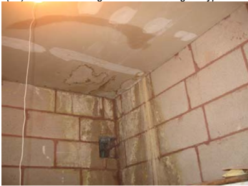
(19) Elevator equipment room – water damage- 7596
