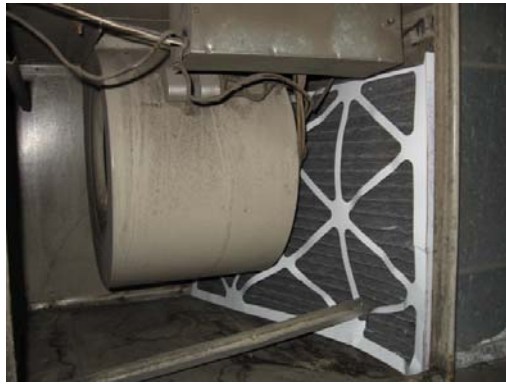
(18) HVAC – filter – typical
