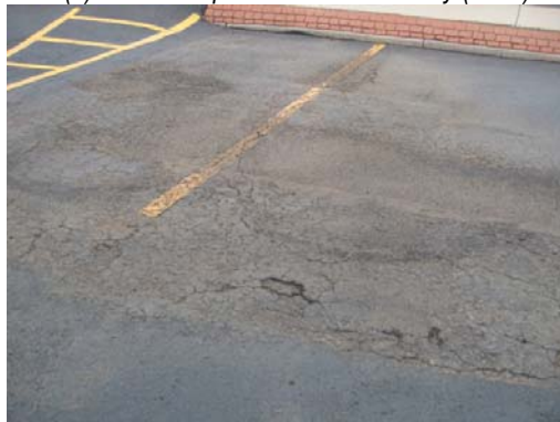
(6) Parking lot irregular cracking/pothole
