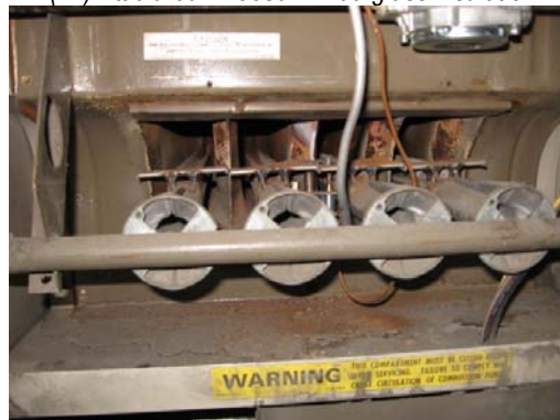
(16) Furnace unit with rust deterioration – typical
