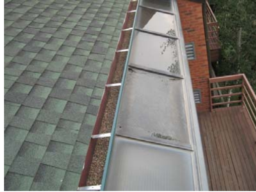
(10) Broken atrium glass 7595 304
