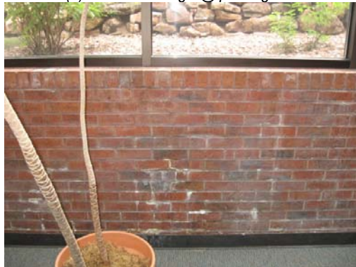
(4) Mineral deposit on brick masonry (7596)
