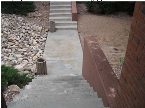
(15) Center egress stairways – no hand rail
