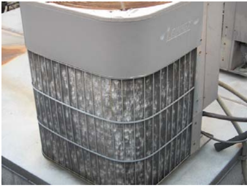
(17) A/C condensing coil – hail damage – typical
