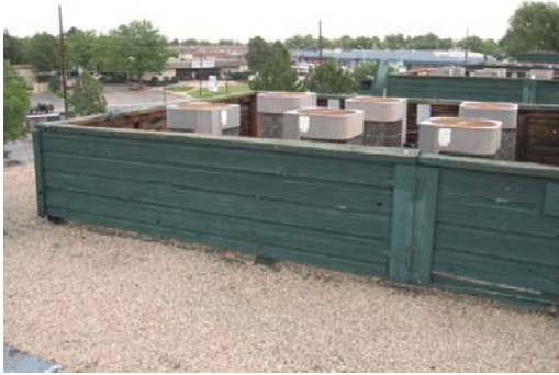
(9) Flat roof/equipment enclosure – deterioration
