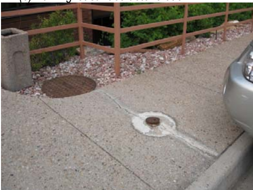
(7) Water main valve @ 7596 trip-hazard
