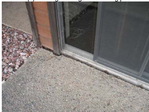
(8) Patio settlement @ rear – typical
