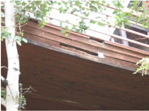
(13) Deteriorated cedar siding @ 3 rd level deck
